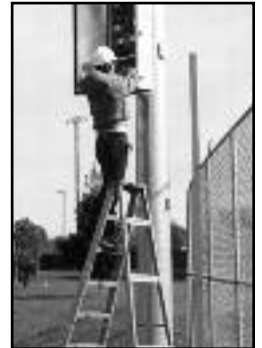
Having major electrical components accessible at ground level avoids hiring a $100 crane to replace a $1 fuse.
