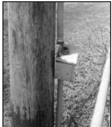
Twisting of this pole caused electrical conduit to separate, exposing wiring.
